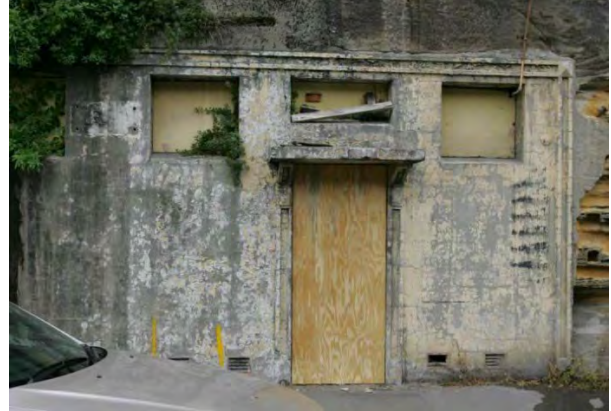
Condition 5 – Very Poor
